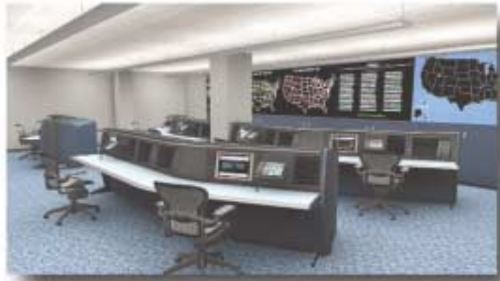
The Building Operations Command Center (BOCC) is a sophisticated, wall-to-wall monitoring system with around-the-clock personnel overseeing all building functions.
