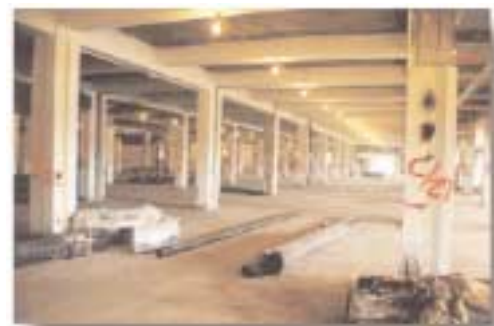
During the demolition and abatement program, everything was removed from Wedge 1, with 70% of the 83 million pounds of debris recycled.
