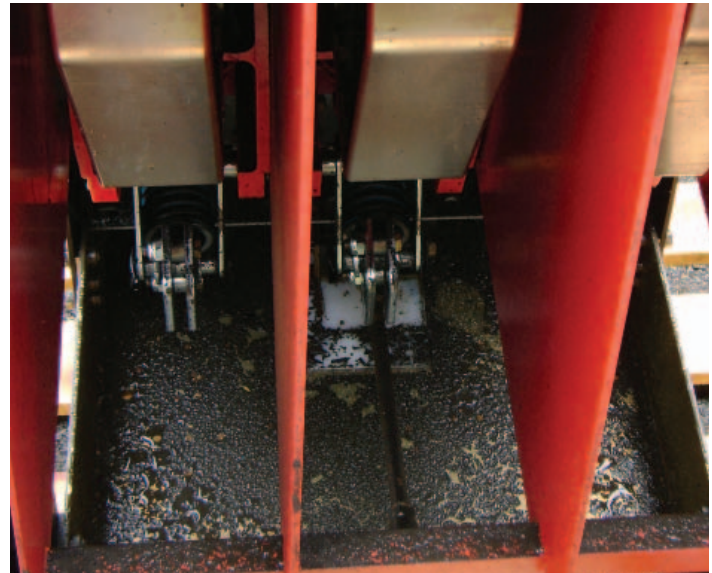
Water-damaged generating plant equipment
