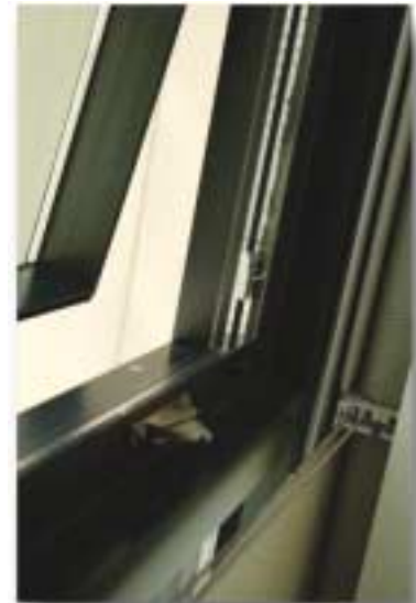
To avoid losing treated air, window contacts were installed, shutting down air to the room when windows are open.
