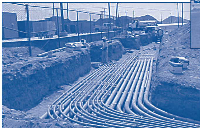
The project included a 7,200-square-foot turbine hall, a 3-mile high-pressure natural gas fuel line, and connections to the electrical substation feeding critical base electricity loads.
